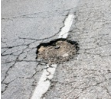
Figure 10: Typical small pothole with missing pavement.
