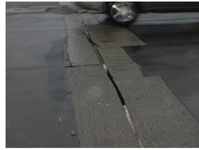
Figure 12: Borderline expansion joint, on a high-speed bridge. This generated a pothole detection.
